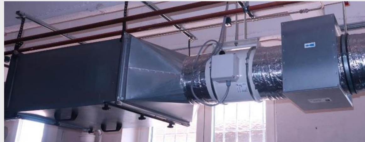
Fig. 12: Air fine filter, tube fan and air pre-filter of the exhaust air system
